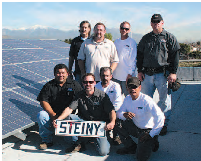
Los Angeles Local 11 members installed a rooftop solar array at a Steiny and Company Inc. warehouse. From left, back row standing, are: Casey Britt, Mark Jacqmin, Dion Mau, Roy Cheaney; front row, Dave Mojica, Wayne Tesoriero, John Garduno and Jose Peregrina.
