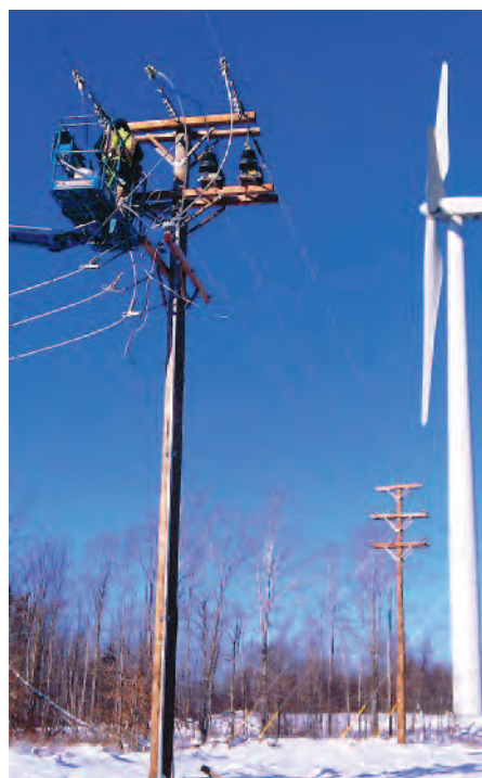
Augusta, ME, Local 1253 members Shane Jordan and Steve Krapf terminate control transformers for signatory contractor Northline Utilities at Stetson Mountain wind farm.
